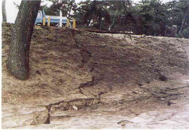
(a) 堤防表のり面の亀裂
