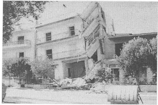
Photo 3 Damage due to pounding, Menidi.
