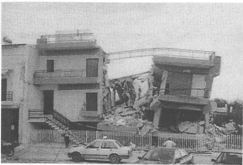
Photo 2 Column failure, due to the short-column effect, in a 5-story building in Ano Liosia.
