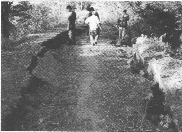
Figure 2: Damaged river dike in San Carlos Lempa
