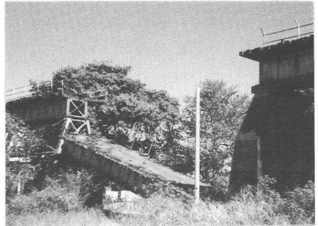
Figure 3: Fallen bridge girder in San Marcos Lempa
