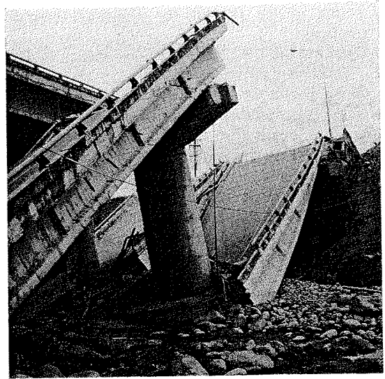
Fig.6 Tilting of Pier P2 towards the bridge axis direction on the DONG-SHYH-bound lane
