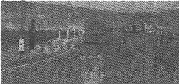
Figure 18: Settlement of bridge approach and cracking of road. Only one lane is open for traffic (looking in southbound direction).
