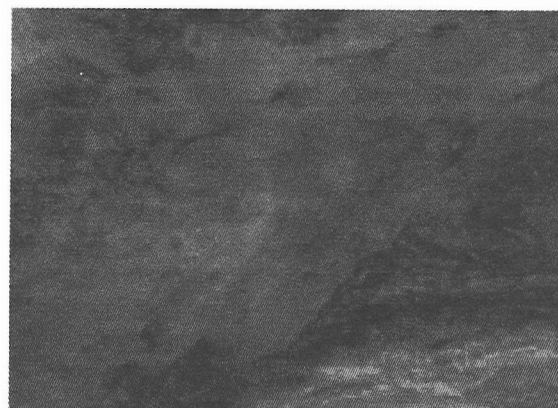
Figure 3: A thrust fault with striations at the northern embankment of Rudramata Bridge (picture towards north) 20km north of Bhuj
