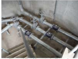
Pipes and Flow Meters in the Elevated Tank
