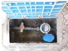
Water Meter (Installed at 4,767 households)
