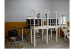
Chlorine Dissolution and Dosing Equipment
