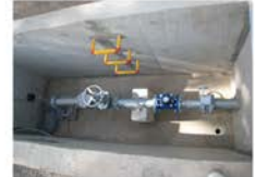
Production Well (56m 3 /h x 4 nos.)
