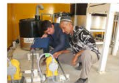
Chlorine Dosing Pump
