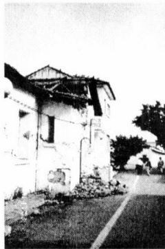
Fig. 3 Severe damage to the structure
