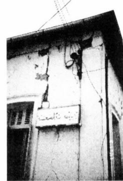
Fig. 4 Severe cracks in walls
