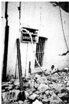
Fig. 2 Damage to emergency wing
